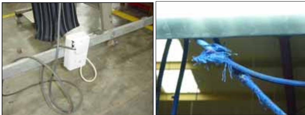
Pictures 14 and 15: A broken electrical socket and frayed electrical cable.
