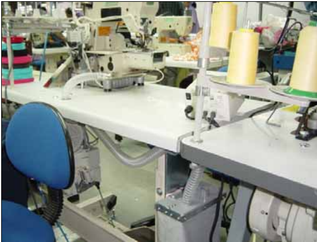
Picture 28: Local exhaust ventilation tubes sucking the dust away from the sewing machine into a waste reservoir which is emptied daily. Note that the suction tubes are placed as close as possible to the source of the hazard.
