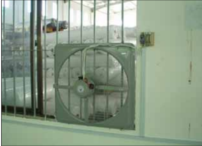
Picture 27: This fan is blowing directly into rolls of material which inhibits the most efficient flow of air. Also look at the electric wiring.
