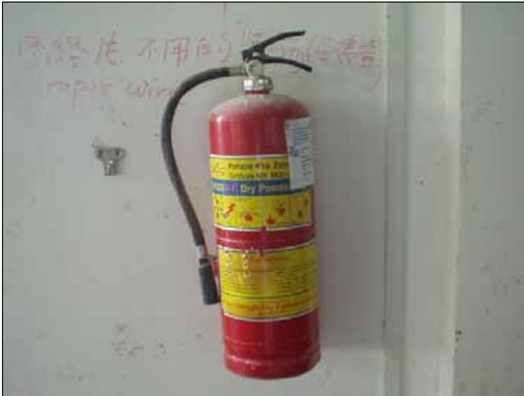
Picture 54: Here is a dry powder extinguisher suitable for type B and C fires as it says on the side of the cylinder. Look at the state of the extinguisher, covered with dust. It is difficult to tell from the dial at the top if it is still operational or needs servicing. Note that there are no signs to clearly show its presence.
