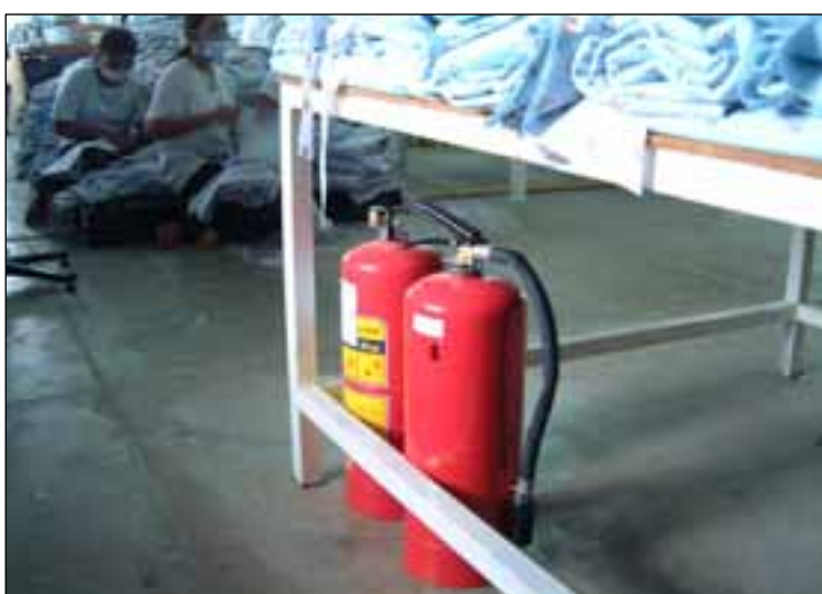
Pictures 57: A blocked extinguisher, how are you to reach it in case of fire? Two extinguishers hidden under a workbench.
