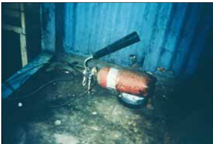
Picture 55: A fire extinguisher that is in an unsafe condition. It will never work and workers would be best advised not to touch it.
