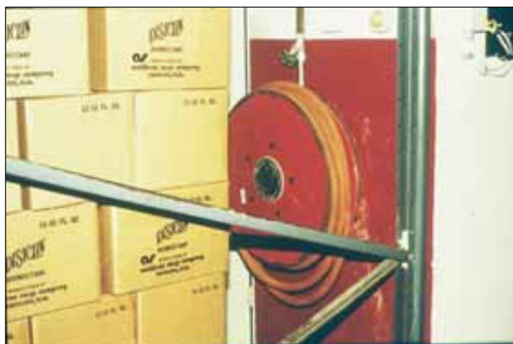
Picture 56: A blocked fire hose/reel. How are workers supposed to reach it in the case of a fire?
